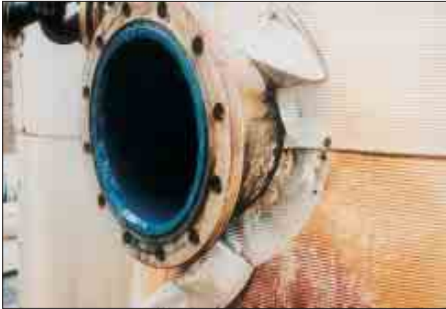
Picture 1 Entrance of CO 2 installation
