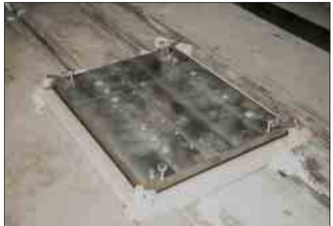
Picture 3 Underfilling of a steel plate
